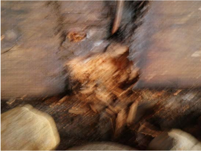
Woods sill – significant rot
