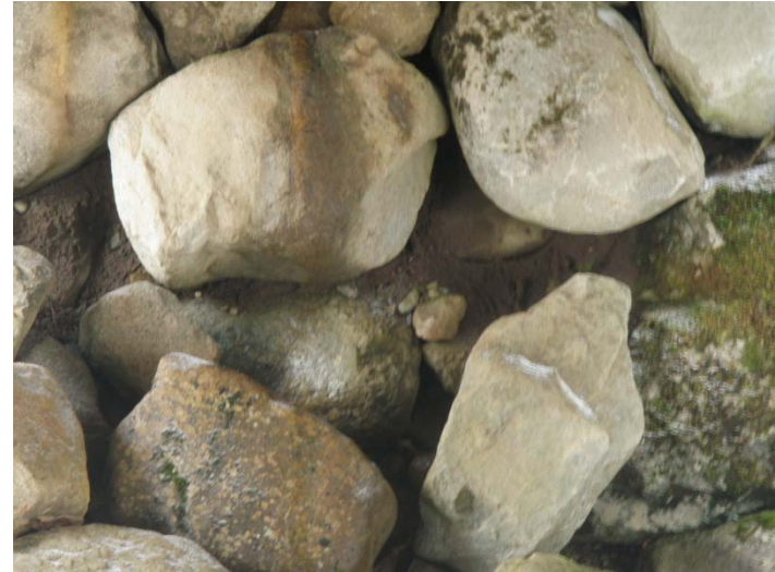
Town riprap undermined
