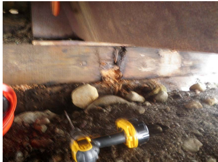
Woods sill – significant rot
