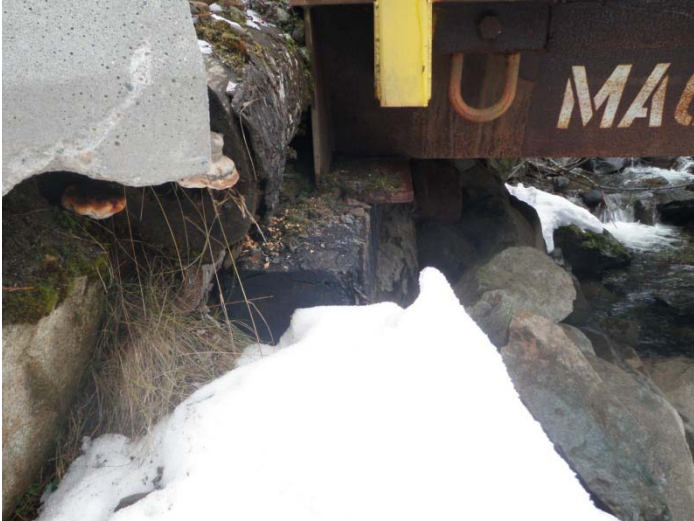
Town bearing plate does not sit completely on sill
