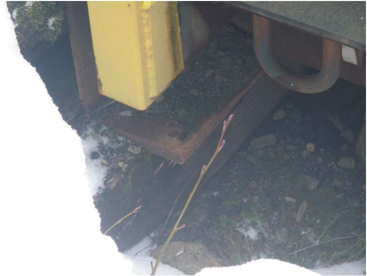
Woods bearing does not sit entirely on sill
